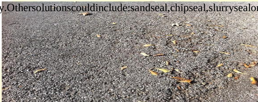
Fig. Raveling(very porous asphalt)
