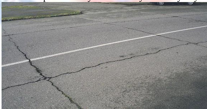
Fig. Joint Reflection Cracks
