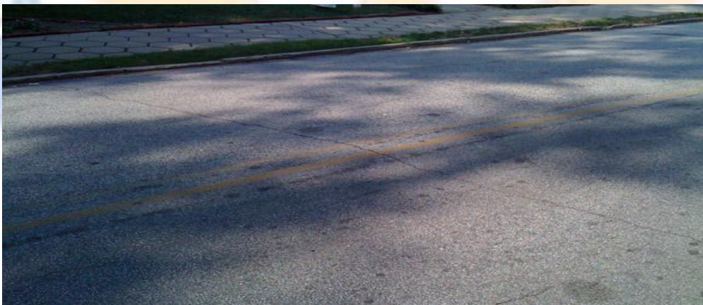
Fig. Transverse Cracking
